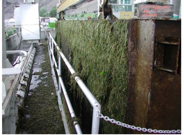
Figure 11b. Top edge of screen that was pulled from the intake valve.
