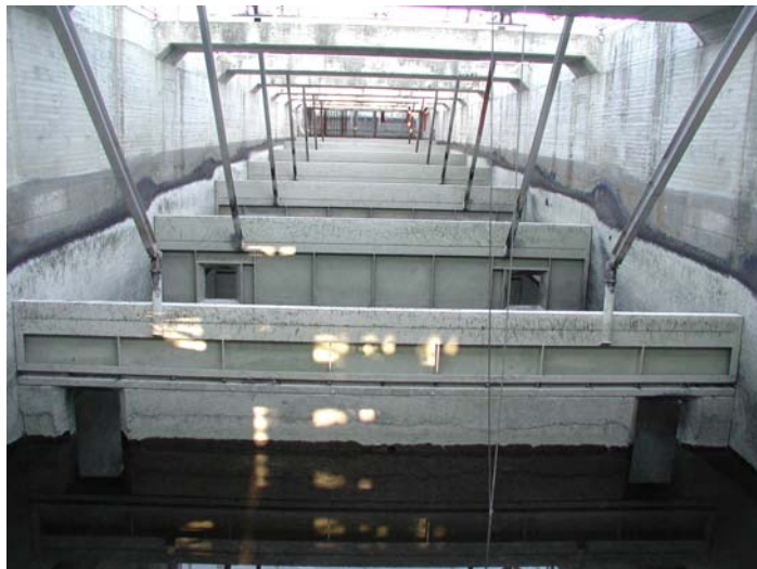
Figure 4b. Tilting weir gates during the winter maintenance period when ladder was being dewatered in 2003.
