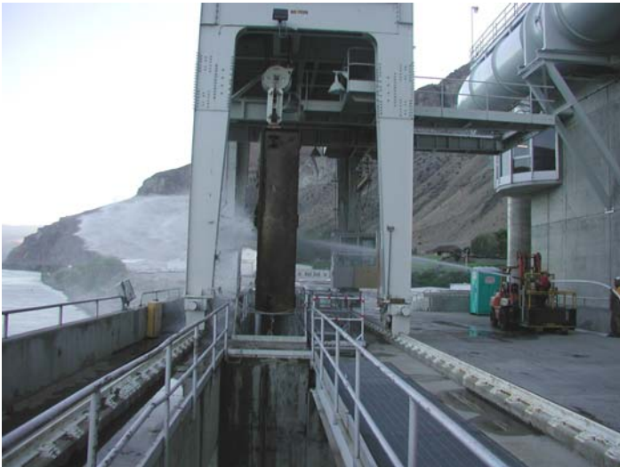
Figure 11c. Crane holds screen in place while project personnel hose grasses from screen.
