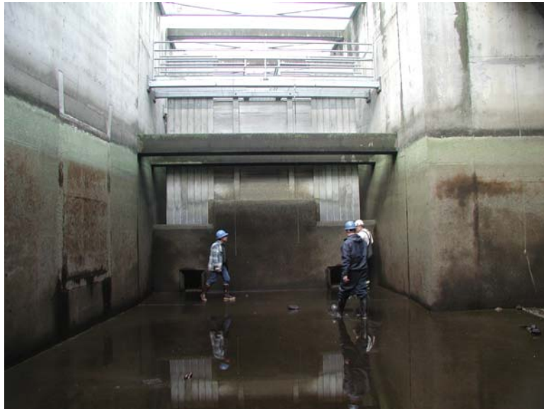
Figure 7b. These two pictures show the poorly lighted area that should lead adult fish from the North shore fishway to this channel that connects to the North powerhouse channel. These lights do not appear to have good passage conditions for fish that enter the North shore and then pass through this lighted tunnel/channel to the North powerhouse area. The same condition would be in service at Little Goose Dam.
