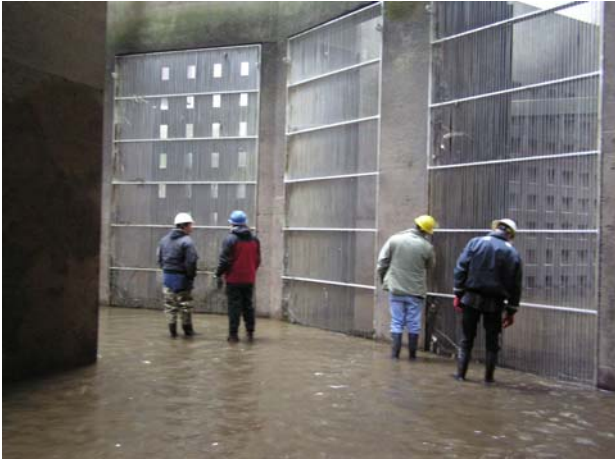
Figure 10a. Photograph taken during 2005 winter Maintenance season showing clean AWSs at the Right Bank fishway at Rock Island new powerhouse.
