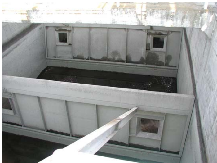
Figure 4a. Tilting weirs at exit from OR shore fish ladder when dewatered for winter maintenance 2003.
