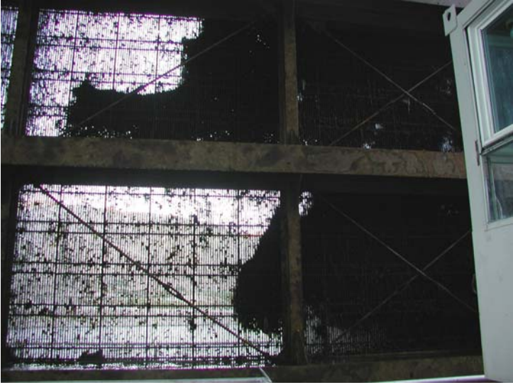
Figure 11a. Photograph depicts pump intake screens with amounts of grasses, resulting in shutdown of the fish pumps until the screens were cleaned.
